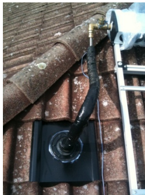
Example of roof duct
